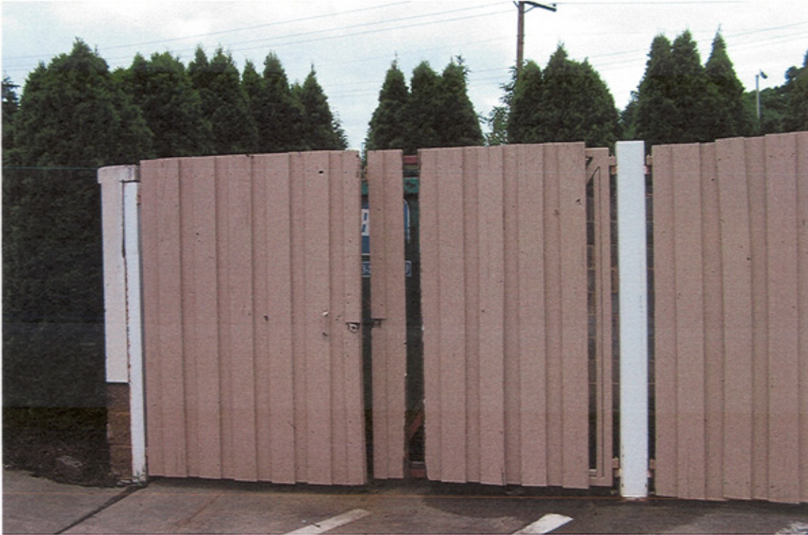
PHOTO 8: Broken and missing boards to the trash enclosure do not fully screen this use.
