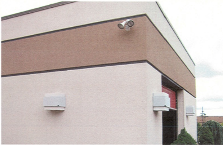
PHOTO 2: One double mounted directional fixture and three wall mounted fixtures can be seen here on the front corner of the car wash.
