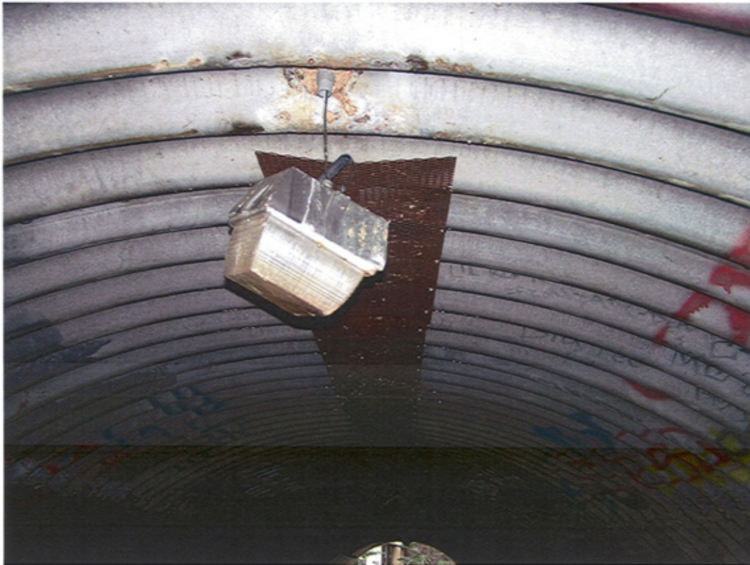
An example of a broken lighting fixture
