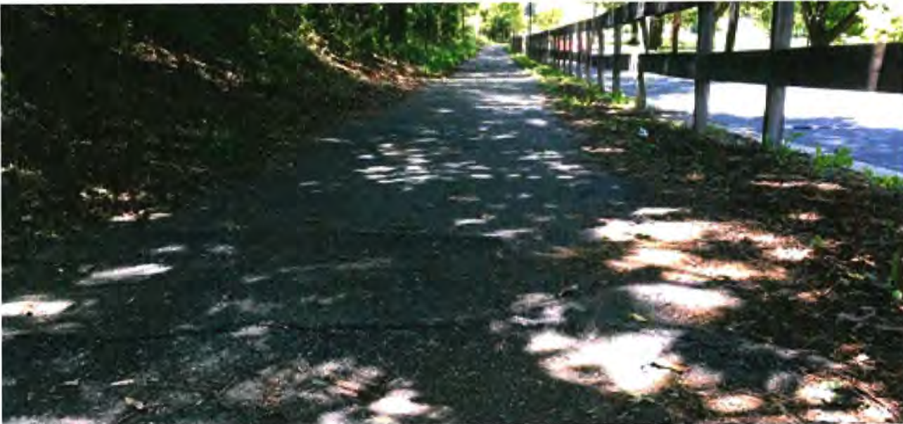
Pavement cracking is common on sidepaths
