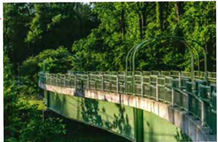
Rock Creek Trail Bridge over Veirs Mill Road near the City of Rockville
