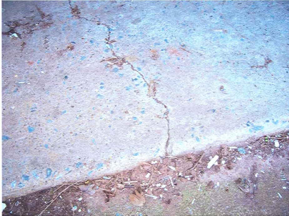
Picture #5: Crack in the concrete garage slab of the historic garage-Maintenance/Vehicle storage.
