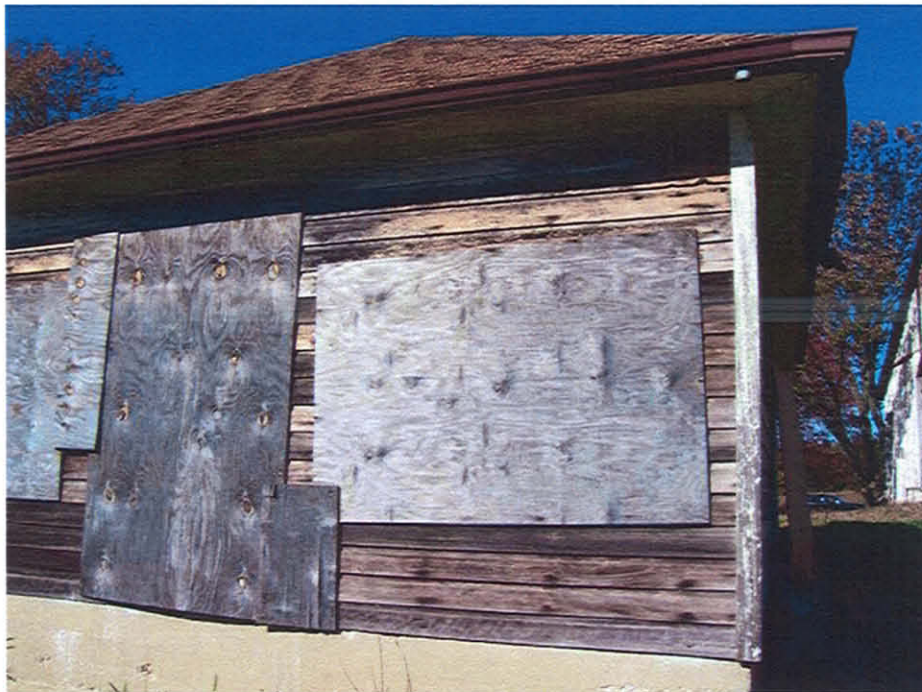
Picture #16: Absence of downspouts in historic farm outbuilding.
