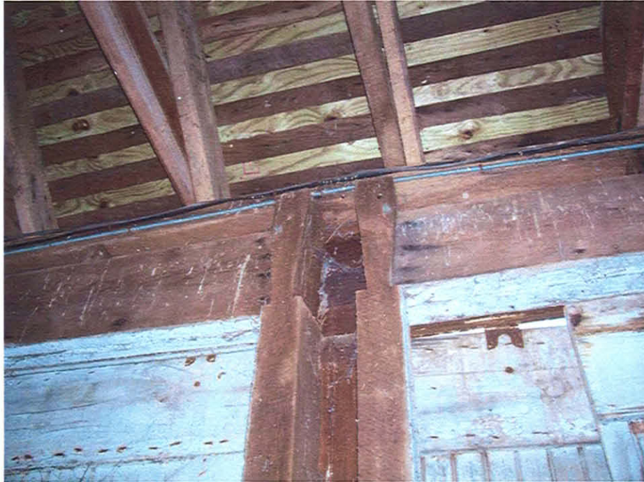
Picture #3: Headers over garage door openings and supporting 4x6 wood posts in the historic garage-Maintenance/Vehicle storage. No hurricane ties at ends of roof rafters.
