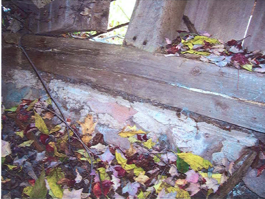
Picture #9: Damaged stone foundation on the south side of the historic barn. Super-Structure is on the verge of collapsing
