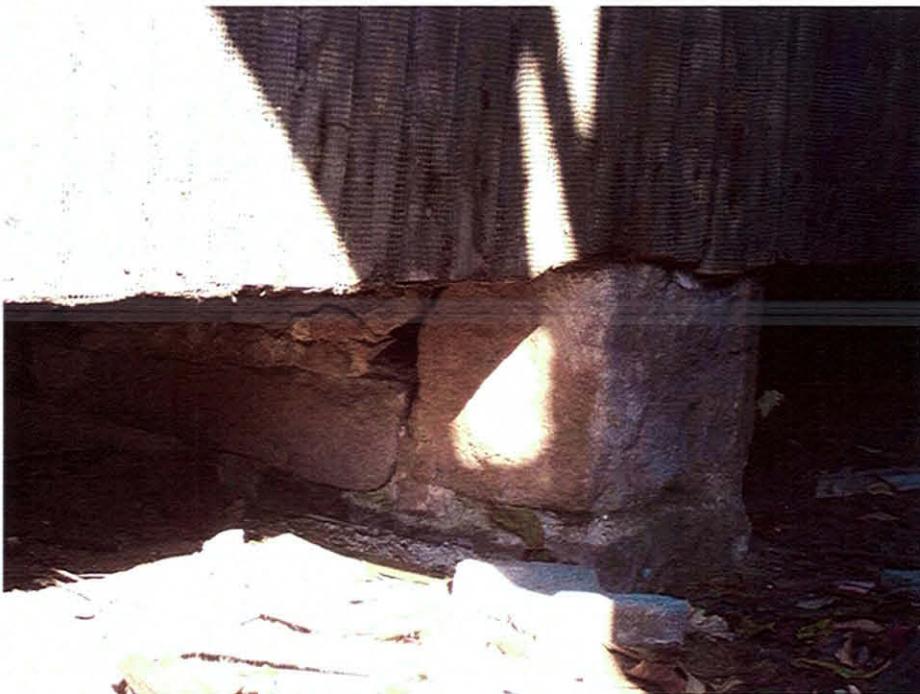
Picture #10: Individual stone piers in the historic barn are in acceptable conditions.
