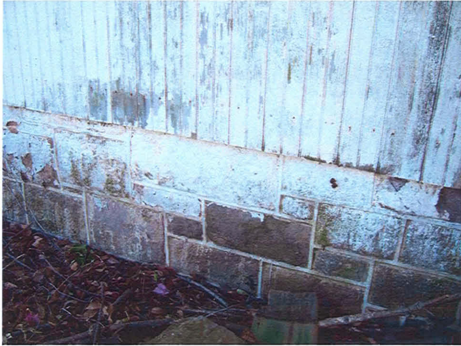
Picture #11: Stone foundation at north side of the historic barn is in acceptable conditions.
