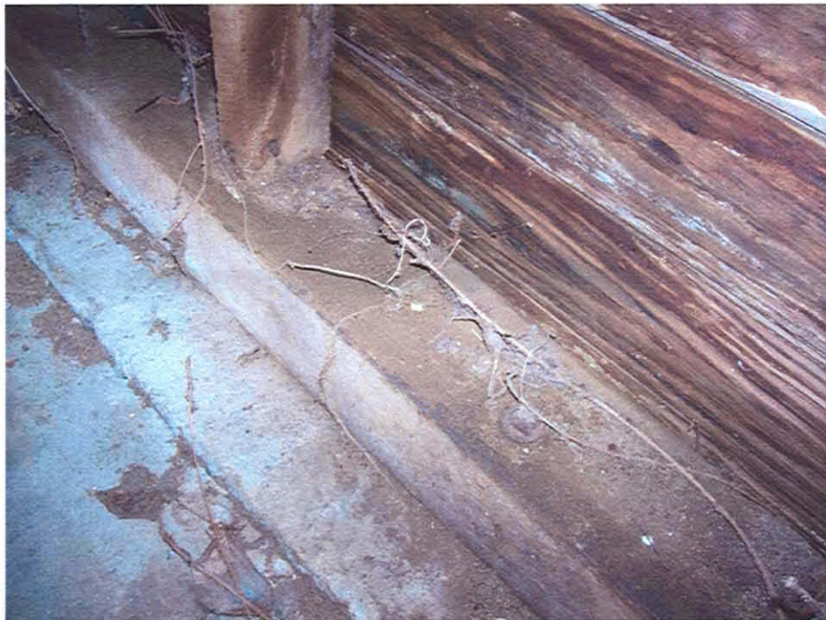
Picture #4: Continuous 4x6 sill plate at perimeter of the historic garage-Maintenance/Vehicle storage. 1/2" diameter anchor is visible in the picture.
