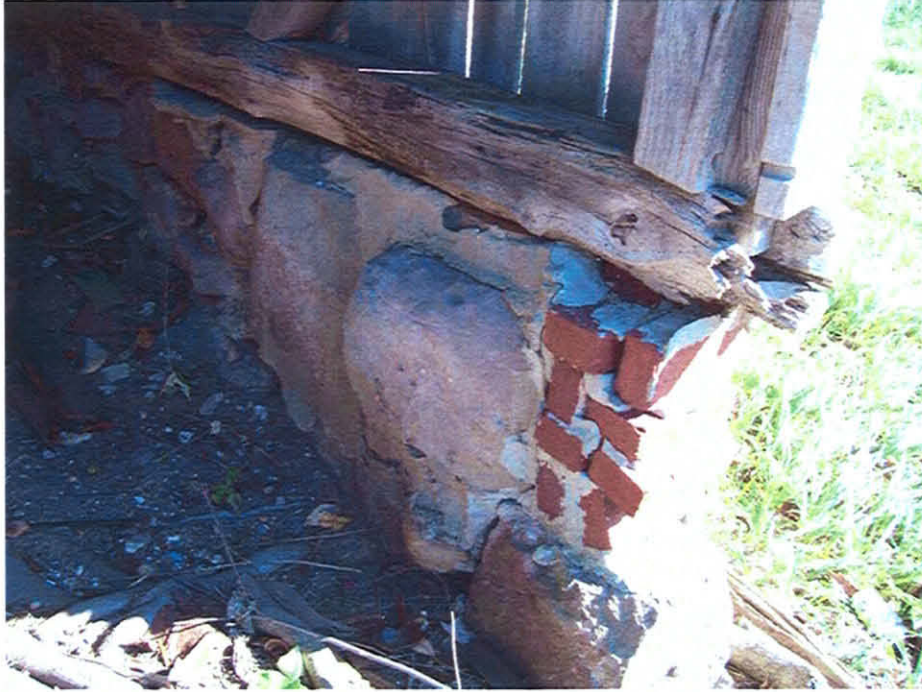
Picture #7: Damaged stone foundation on the south side of the historic barn.
