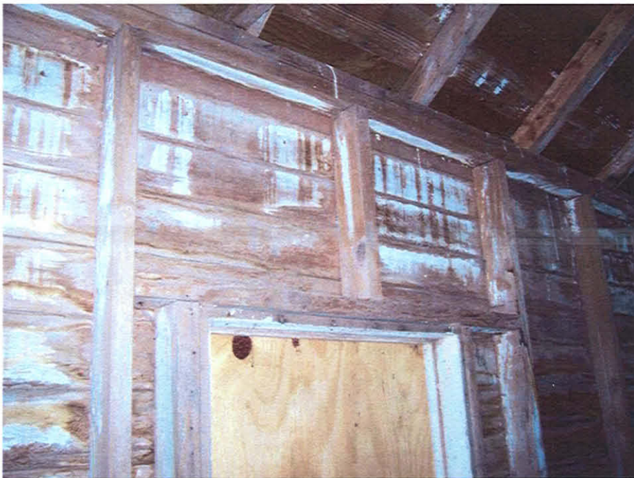
Picture #14: Historic farm outbuilding. No hurricane ties at rafter ends and no headers over openings
