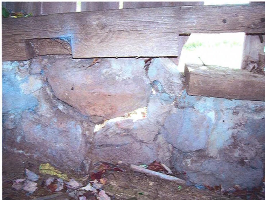
Picture #8: Damaged stone foundation on the south side of the historic barn.
