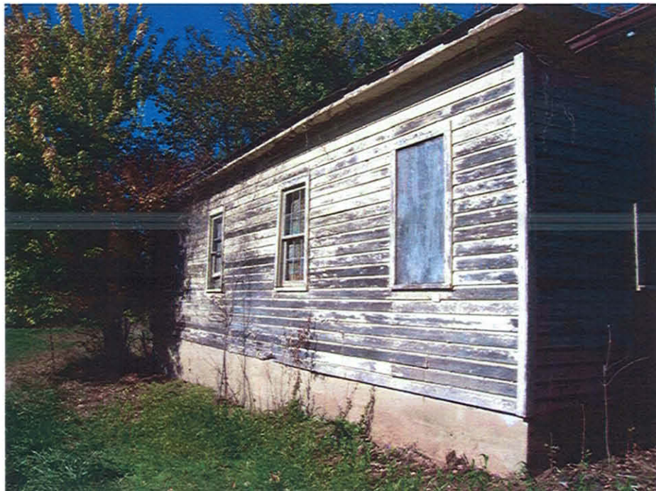
Picture #6: Deterioration of siding at the historic garage-Maintenance/Vehicle storage.
