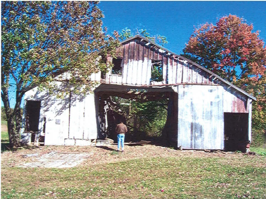
Picture #12: Super-structure of the historic barn is on the verge of collapsing.
