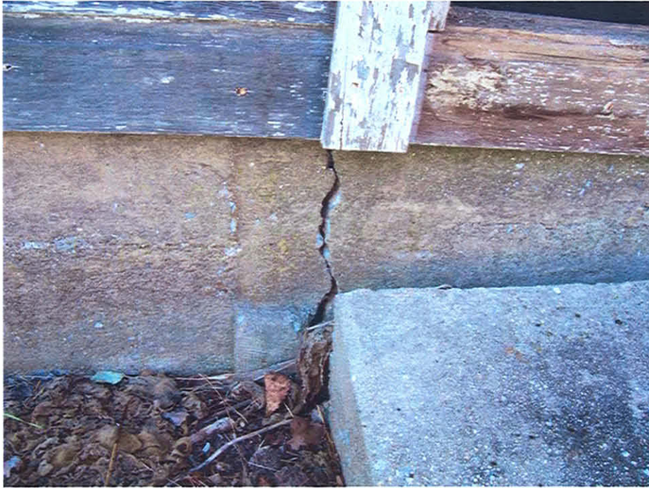
Picture #15: Major structural crack on the foundation wall of the historic farm outbuilding
