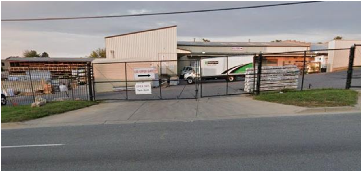
This fencing of this gated entrance along Snouffer School Road is located too close to the roadway as it does not allow for the stacking of at least two vehicles outside of the public right of way.
