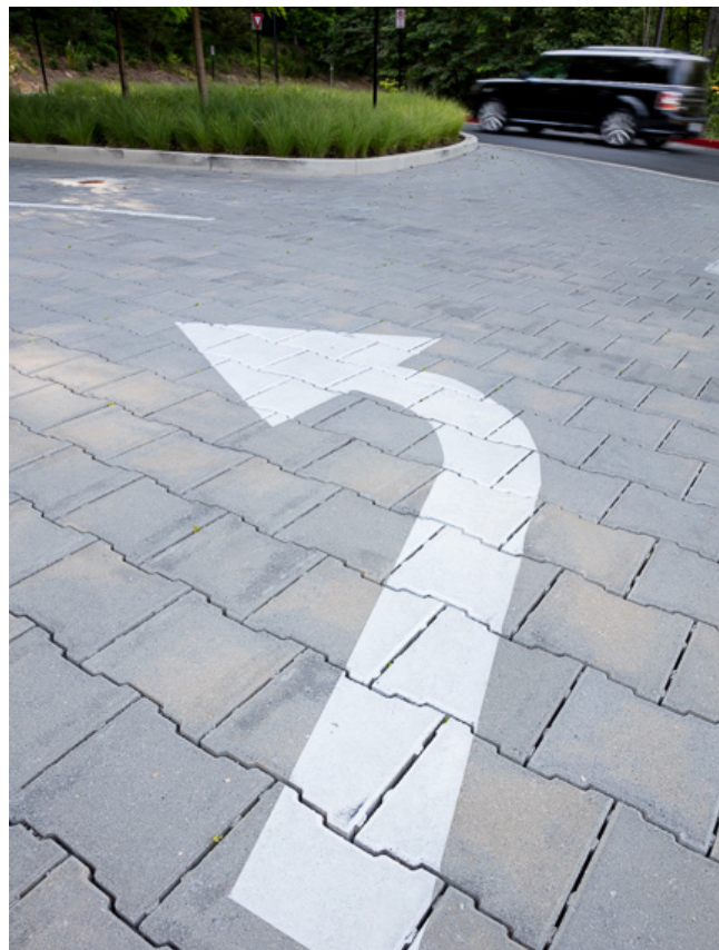
The parking lot at the Brookside Gardens Visitor Center uses permeable interlocking pavers for the parking spaces (Montgomery Parks).
