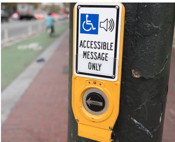
An accessible pedestrian signal reads "Accessible Message Only" and has a confirmation light. Photo Credit: SFMTA
