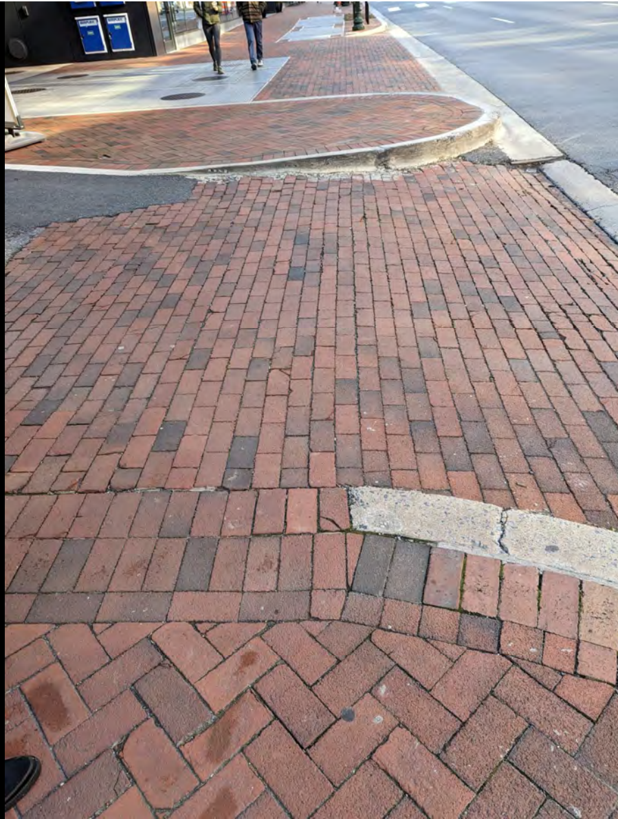
Wisconsin Ave. Driveway curbs present tripping hazard and wheelchair obstacle
