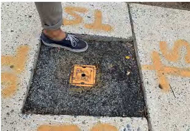
A poorly filled utility cut in the sidewalk. Shoe for scale.
