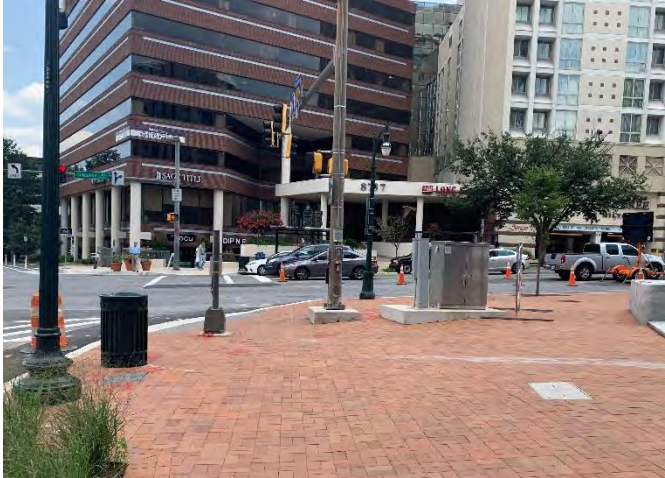
Traffic signal control cabinet in the sidewalk in downtown Silver Spring.
