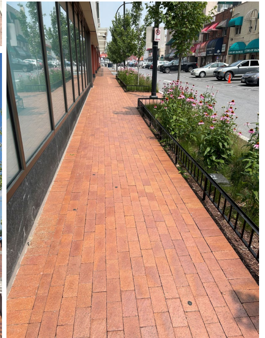
Existing pavement conditions in downtown Wheaton
