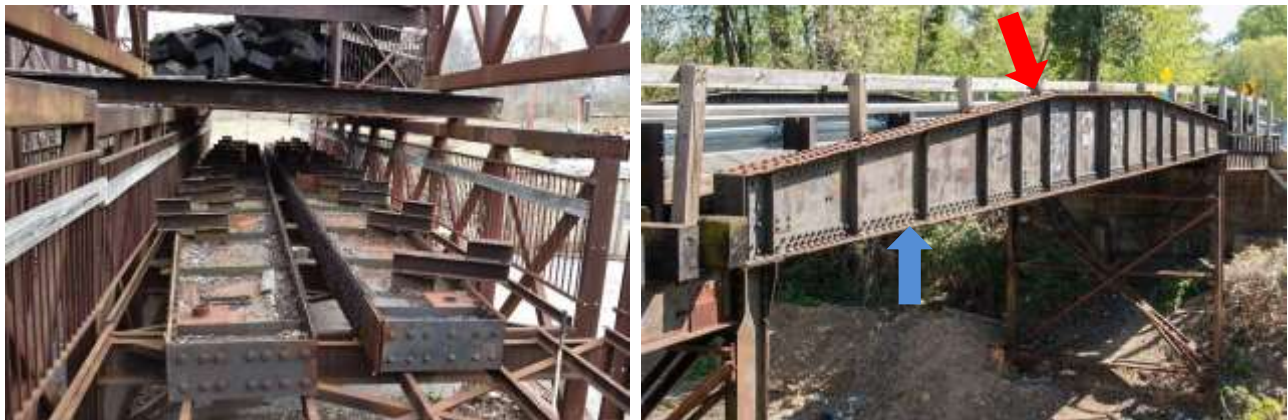
Figure 3 (Right): Overall picture of the two plate girders lying flat at the storage facility in Silver Springs, Maryland. (Photo: EverGreene (March 22, 2023))
