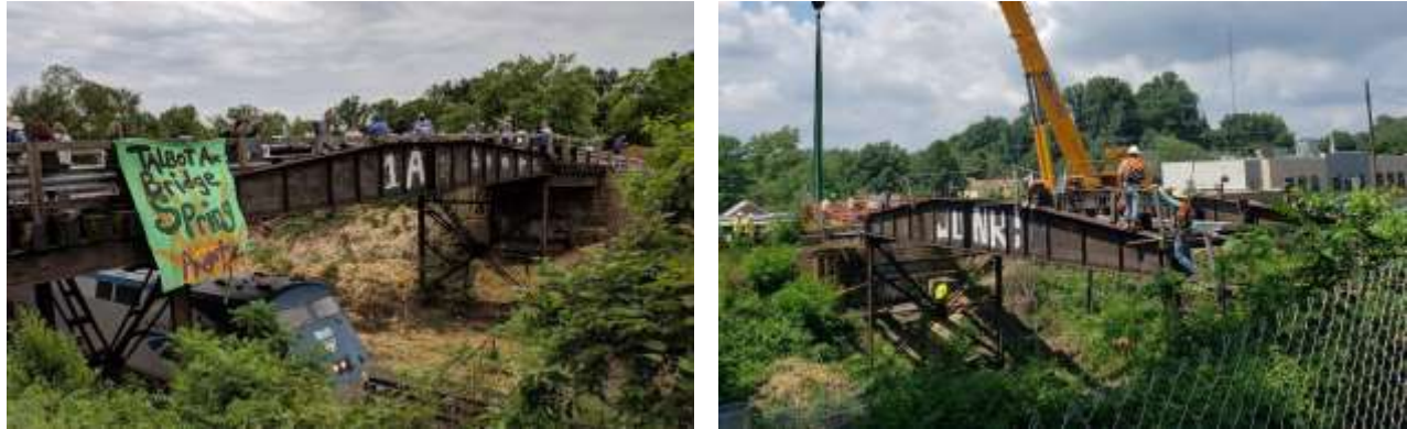
Figure 9 and 10:: Figures 11 (Left) and 12 (Right) are of the Talbot Avenue Bridge in 2019 during the removal. Notes the heavy graffiti on both the North (left) and South (right) sides. (Photos: Talbot Avenue Bridge Facebook Page (2019))
