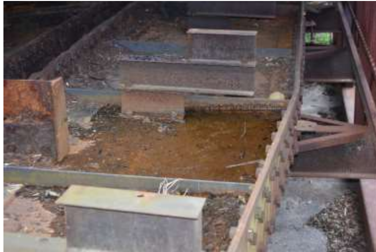
Figure 17: Detail of Bay 5 where water is collecting on the west side of the horizontal plane. (Photo: EverGreene (March 22, 2023))
