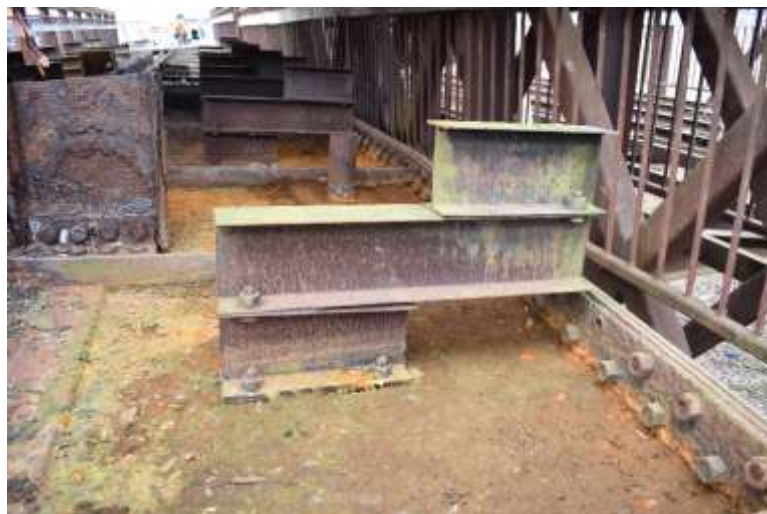
Figure 13: Detail of the guardrail I-beam in Bay 11. Note the bio-growth concentrated on the vertical and skyward facing planes. (Photo: EverGreene (March 22, 2023))
