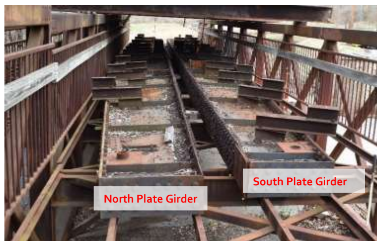
Figure 11: Photograph of the 2023 conditions and orientations of the north and south plate girders. Photograph was taken facing north. The north plate girder is located on the west side of the storage area and the south plate girder is located on the east side. (Photo: EverGreene (March 22, 2023))
