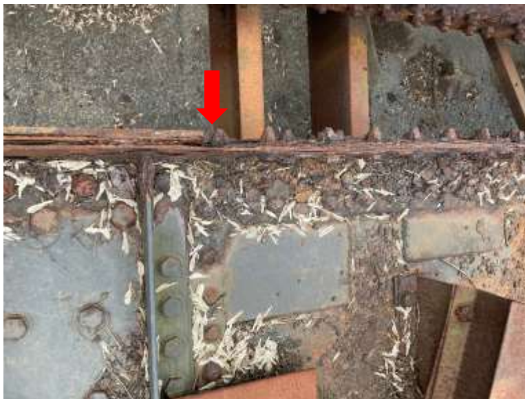
Figure 16: Detail of the lower flange of Bay 1 on the south plate girder. The Red arrow shows where the gusset plate and exploded corrosion are separating from the rest of the flange structure. (Photo: EverGreene (March 22, 2023))
