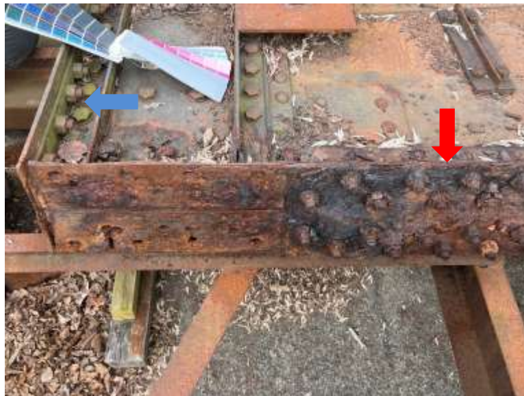
Figure 12: Detail image of Bay 1 of the bottom flange of the north plate girder. The red arrow shows the condition of the corroded flange cover plate and hex bolts and blue arrows shows the area mostly unaffected by the corrosion. (Photo: EverGreene (March 22, 2023))
