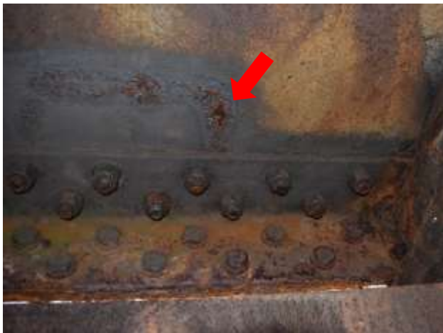
Figure 17: The red arrow shows the weeping or active corrosion found on the underside of the North Plate Girder. (Photo: EverGreene (March 22, 2023))
