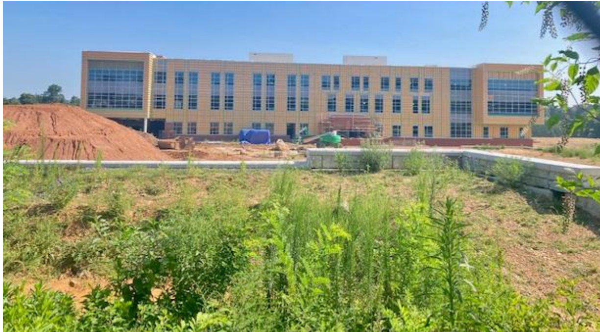
Figure 4: South elevation of new school building (from Cedarwood Drive- Mains HOA- facing north)
