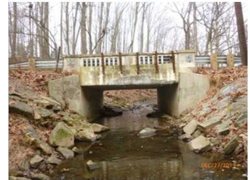
Undersized Bridge Opening
