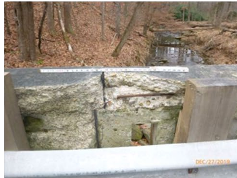
Spalled Concrete Railing
