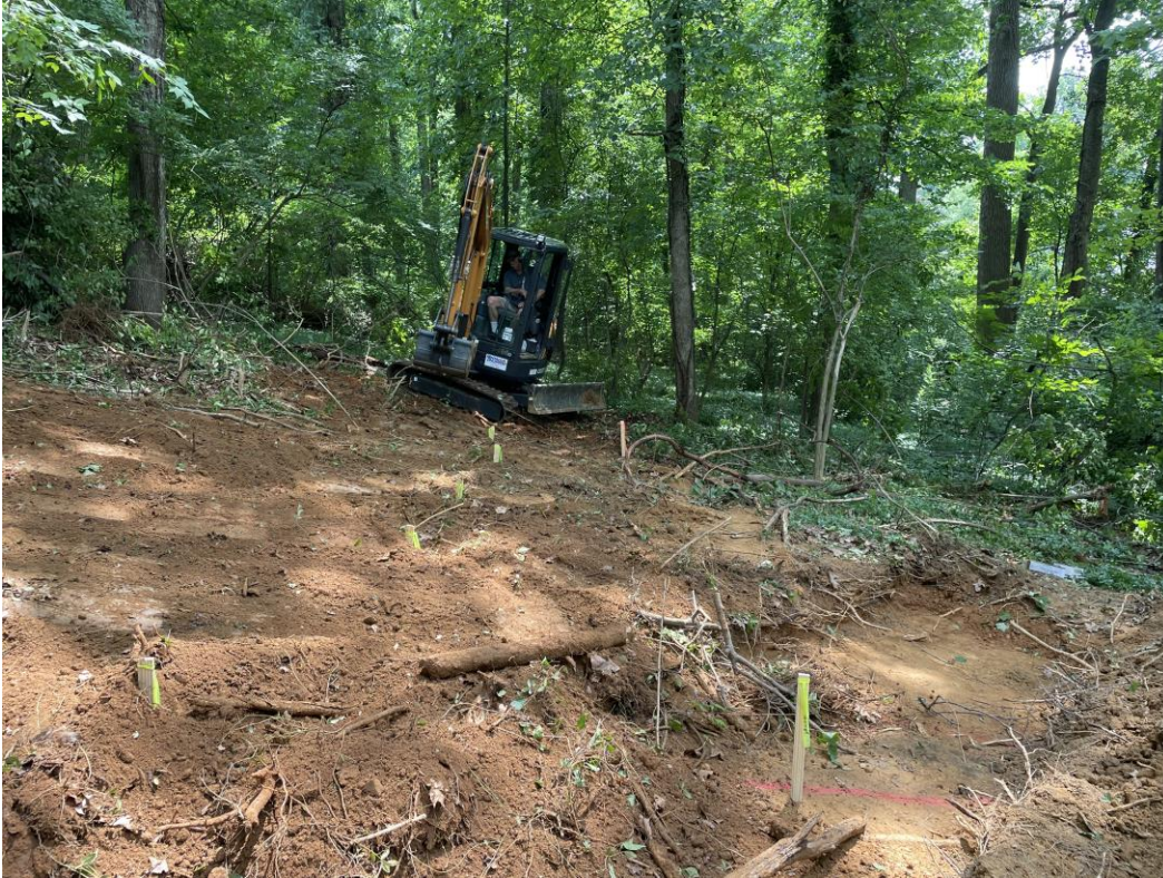
Photo 7: View of trench backfilling at the completion of fieldwork, facing south. Note wooden stakes marking locations for survey.
