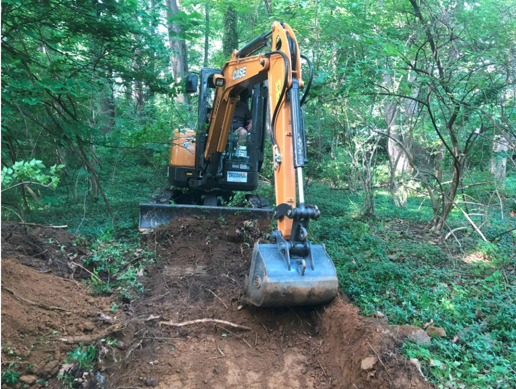
Photo 3: View of mechanical stripping of surface soils within the mapped cemetery area.
