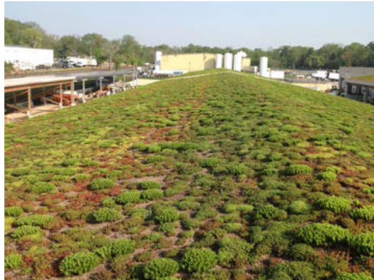
Example: Green Roof on structure at Shady Grove Equipment Maintenance and Operations Center
