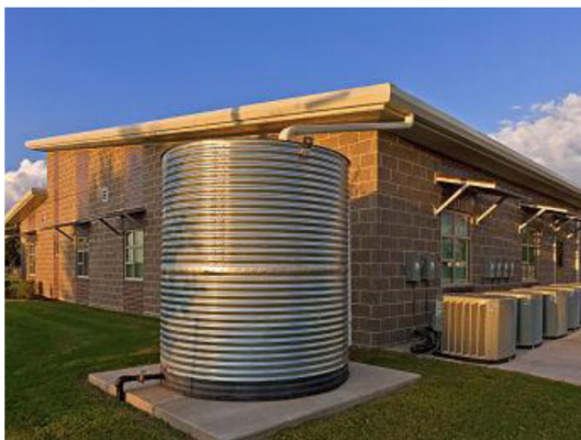
Example above grade cistern
