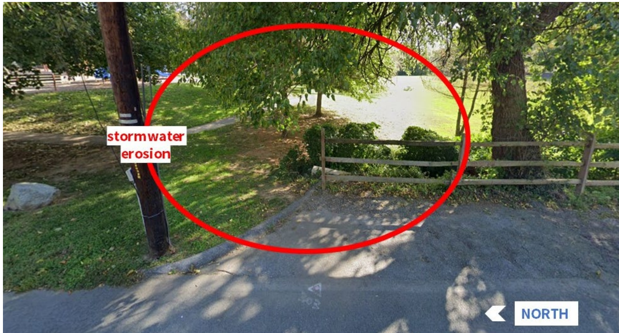
Figure 15: Streetview Image of Existing Asphalt Apron and Erosion at Bullis Local Park
