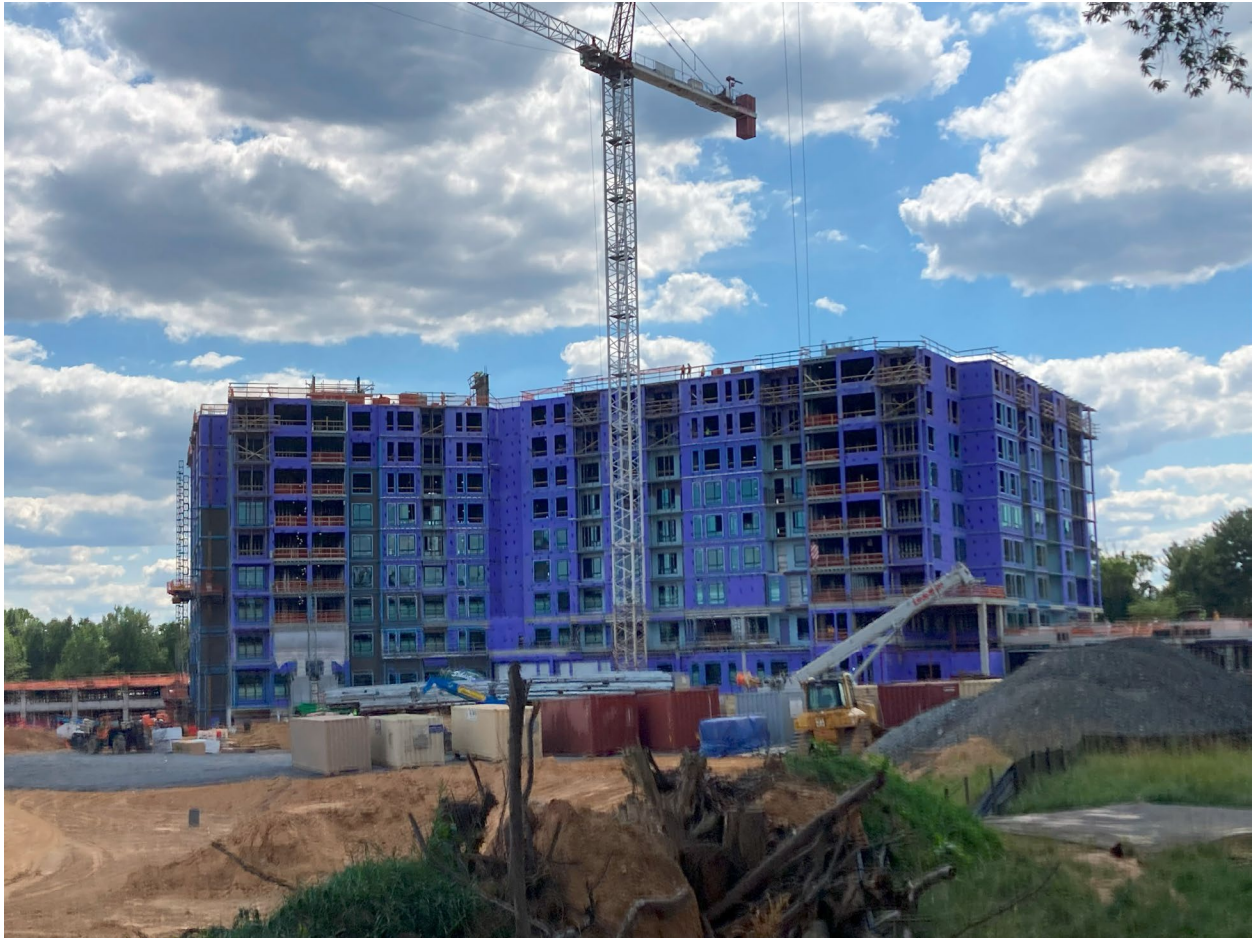
Figure 4 – View of construction progress on the Subject Property, taken in July of 2024
