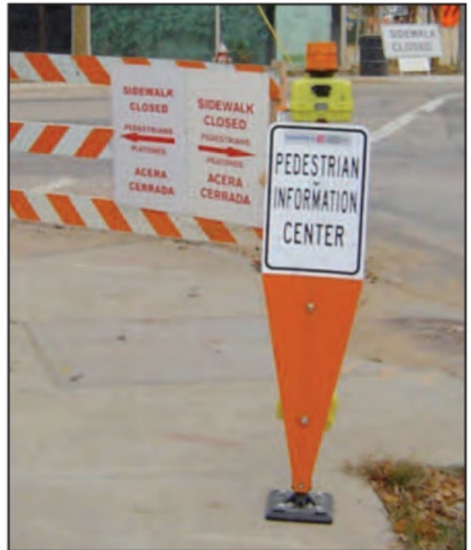
Figure 63: Audible information device in advance of a closed sidewalk (Source: American Traffic Safety Service Assoc. Applying the Americans with Disabilities Act in Work Zones: A Practitioner Guide)
