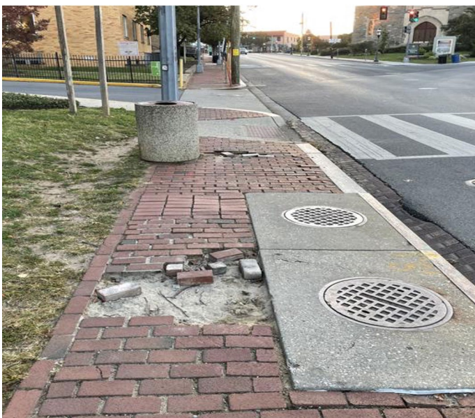
Figure 17: Example of deteriorated brick sidewalk
